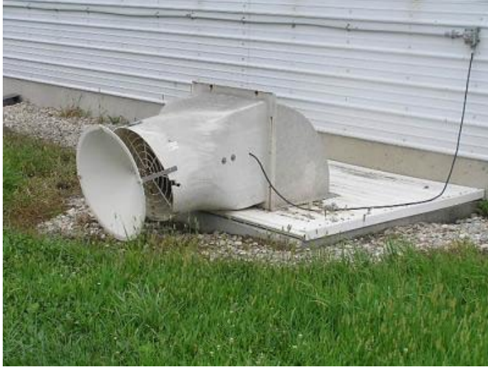
Figure 4 – Image of a typical pit fan located on the outside of a hog barn (AMPAT).
